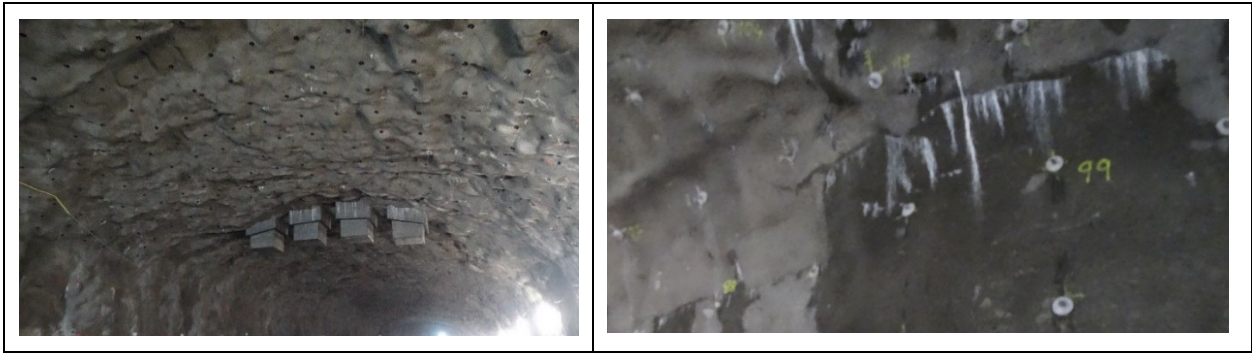
Figure 14. Predominantly wet dark-looking shotcrete (and leaking bolt holes) may be seen when too low pressures and incorrect grout selection is made. It also will not help to delay bolting and have too narrow pillars between large pre-injected tunnel spans in the case of motorways. In the left-hand photo two light-coloured noses are seen in the arch – where shotcrete was able to dry. The wet shotcrete may be assisting groundwater drawdown along the motorway corridor.
