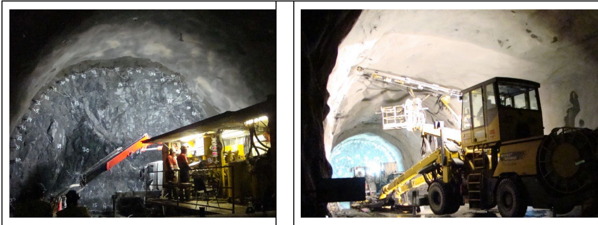
Figure 1. The Bærum Tunnel west of Oslo with systematic pre-grouting of 5km length and 1 to 2 litres/min/100m result with no need for the pre-installed infiltration wells. This project is a good example of the gradual improvement in achievable inflow limits, which has reduced in Norway from about 30litres/min/100m some 40 years ago, to about 10litres/min/100m about 30 years ago, and down to best results of about 1-2litres/min/100m in the last 10 - 20 years. Note the dry shotcrete in the current last 50-60m of this tunnel, in contrast to the occasional small wet patches. Filter-pump discrimination against stable grouts with micro-silica has been shown to cause 'reversal' of the dry/wet shotcrete experience – meaning mostly wet shotcrete and a minimum of dry patches. This is an undesirable and totally unnecessary result.
