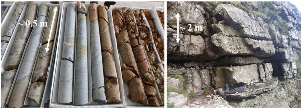
Figure 29 Examples of identification of potential MFC left photo: core drilling indicating contact between sandstone (UCS ~ 100 MPa; low degree of fracturing) and lutite (UCS ~ 15 MPa; highly fractured), right photo: field mapping indicating potential MFC due to blockiness (Macias et al. 2020).
